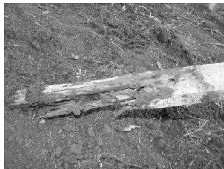
Foto 8: Ataque de termitas Photo 8: Termite attack
